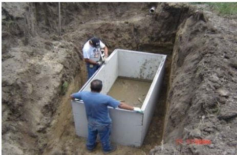
Replacing a septic tank in Martin: Archie Red Owl (back) and Tony Hernandez (front).
